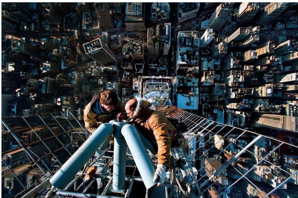
These three guys are working on an antenna high atop the Empire State Building in New York City. One of them took this picture — Submitted by Doug Burkart
